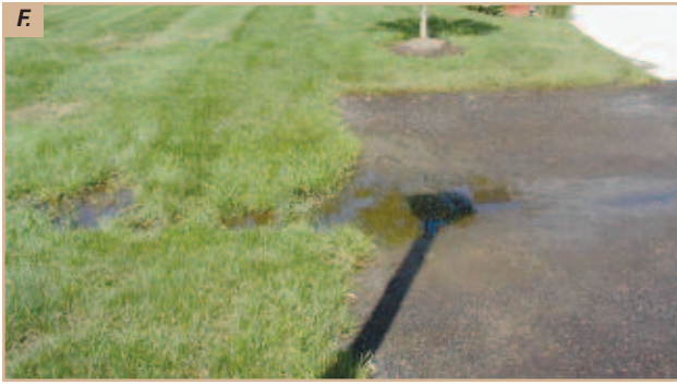
Figure F. Ponding water can deteriorate pavement, resulting in un-maintainable lawn areas while creating an insect breeding environment.
