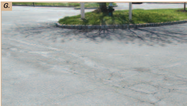
Figure G. Freeze/thaw cycles can cause severe pavement failures especially if cracks are not sealed prior to winter
