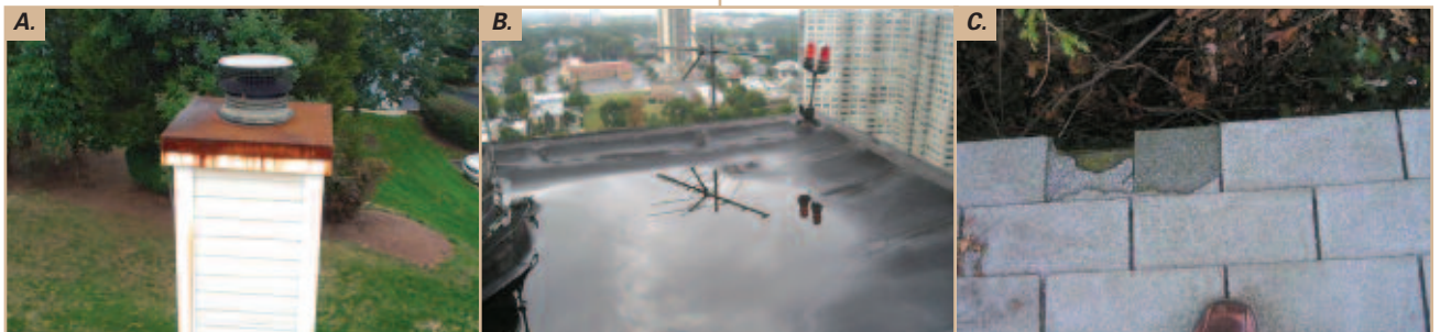
Figure A. Rusting or improper attachment of chimney caps can result in water infiltration into the building. Figure B. Ponding water on a flat roof will likely lead to leaks and structural damage. Figure C. Damaged or missing shingles can lead to water infiltration.
