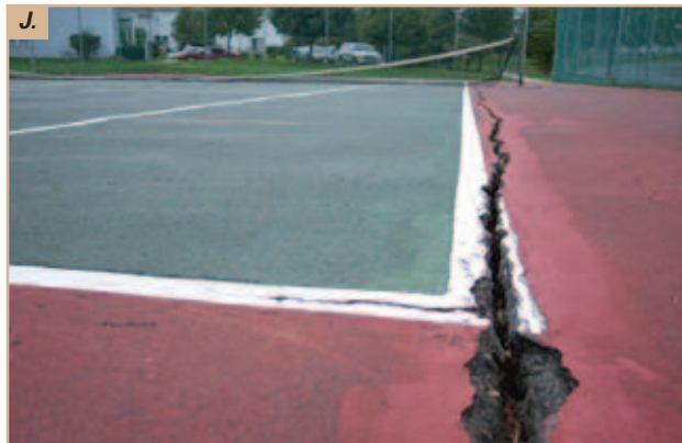
Figure J. Safety concerns for all recreation facilities and tot lots requires focus, attention and timely maintenance.
