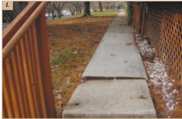
Figure I. Tripping hazards need to be alleviated with concrete replacement.
