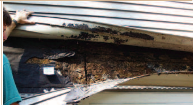
Unfortunately, siding may appear in good condition from the surface, however significant damage may exist behind the product.
