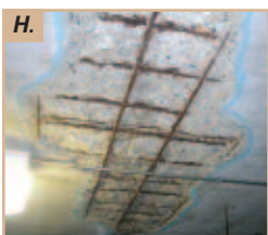
Figure H. Advanced deterioration of a parking structure, areas below and above the structural deterioration are not safe.
