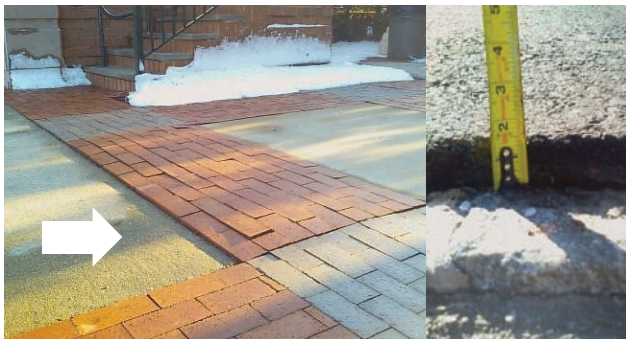
Figure 1 – Example of a Heaving Walkway
